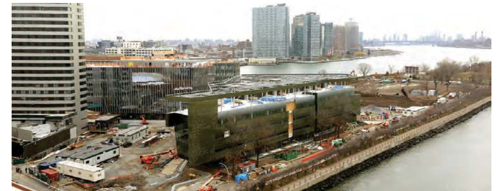
View of construction on Cornell Tech's Roosevelt Island campus from the Queensboro Bridge.
